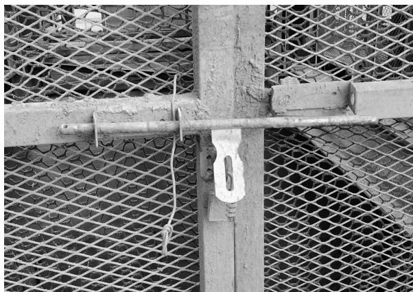
The only thing holding this gate closed was a green netting.
